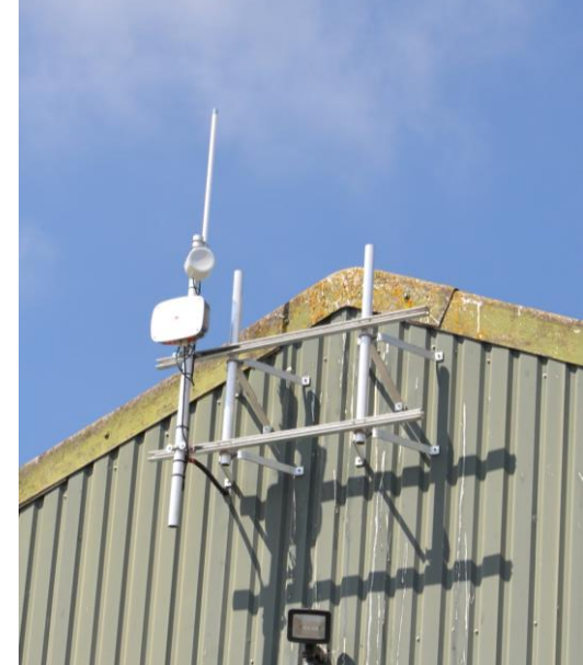
Barn Mounted Base Station
